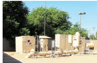
Mesa Pumping Station
